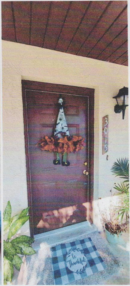
Unprotected non-glazed entry door
