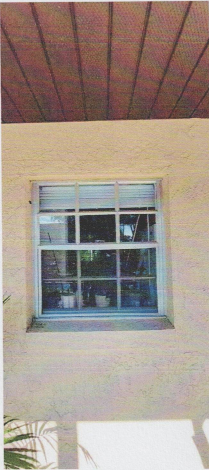
Unprotected glazed opening
